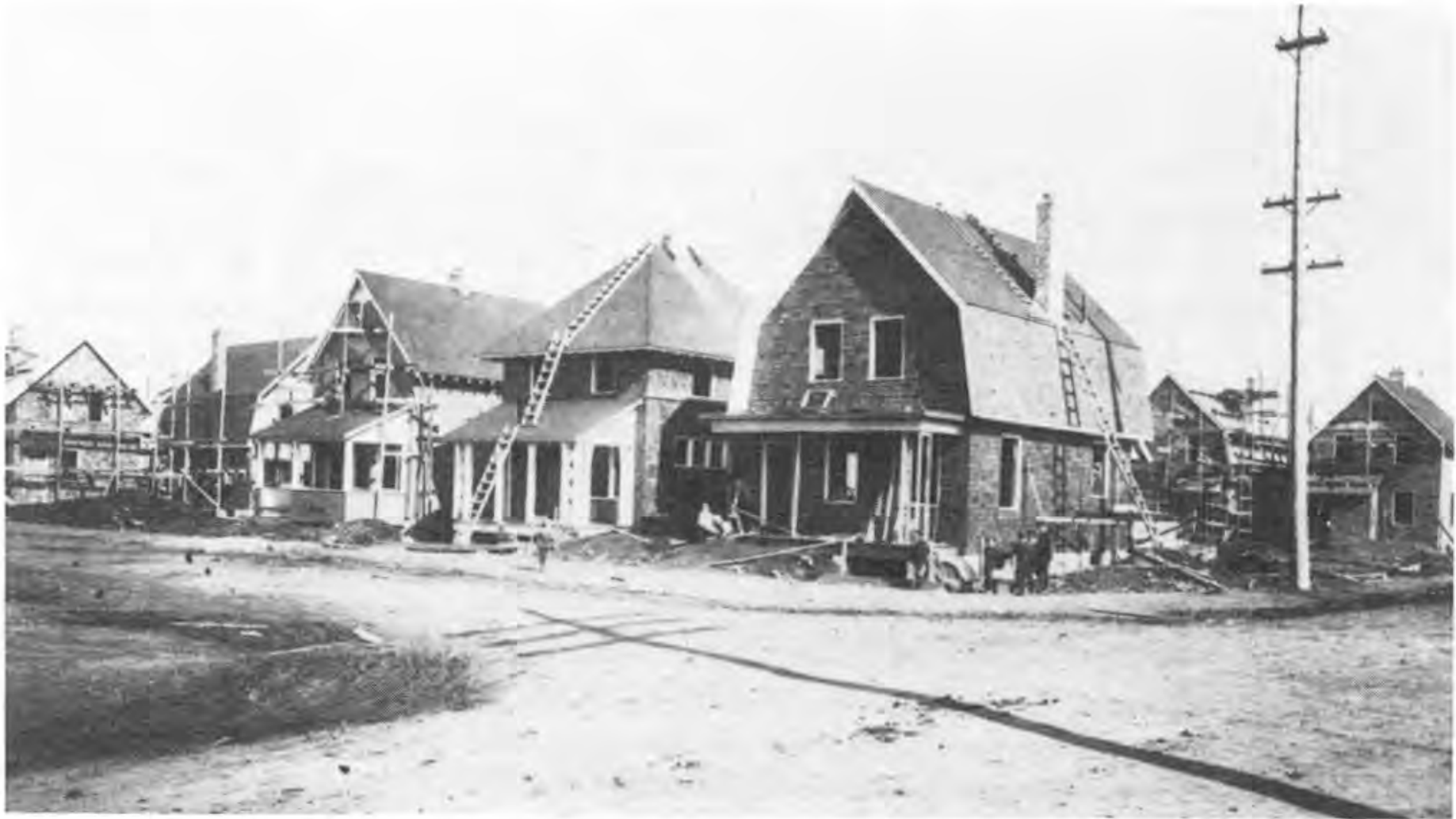
Figure 6. The Highfield subdivision, soon to be owner-occupied, under construction at Robie and West Young streets. (Gauvin & Gentzel, PANS negative N-7042)
